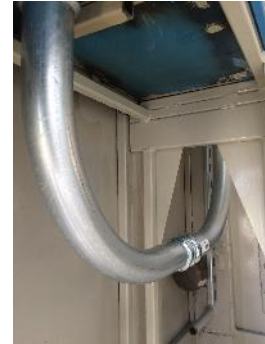
Figure 40. EMP protected conduit
